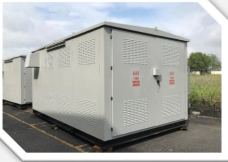
11kV 1000kVA Package Sub-Station (Bioconversion Plant, Ijok)
