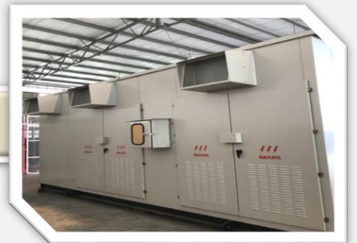
11kV 1500kVA Package Sub-Station with LV MSB (1MW Biogas Power Plant, Kedah)
