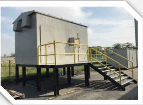
E-House for 33kV GIS Panel, RE Plant (20MW LSS Power Plant, Batu Kawan)
