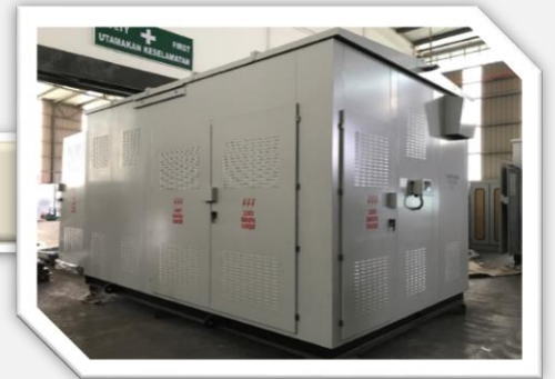
33kV Package Sub-Station with 1600A MSB (30MW LSS Power Plant, Gebeng)
